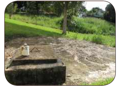
Keep septic tanks sealed.
